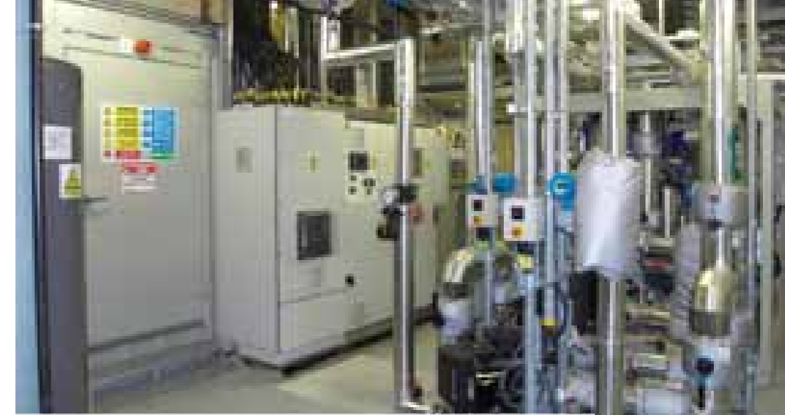
CHP Plant room internal view with engine located within acoustic enclosure
