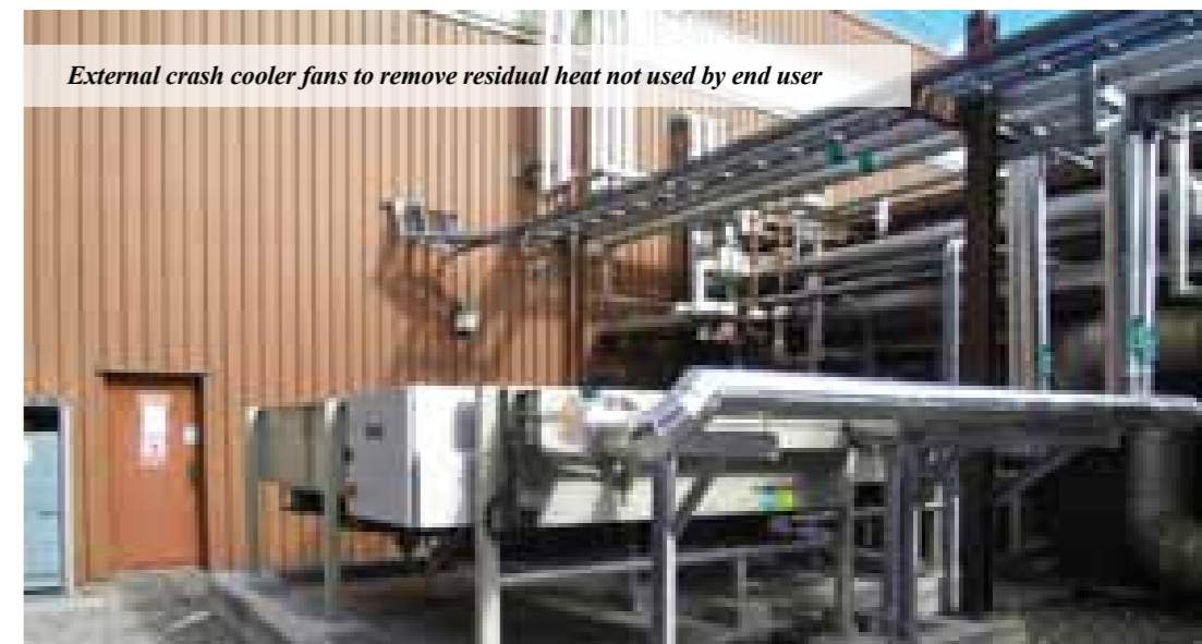
Associated high grade/low grade heat exchangers/pump skids
