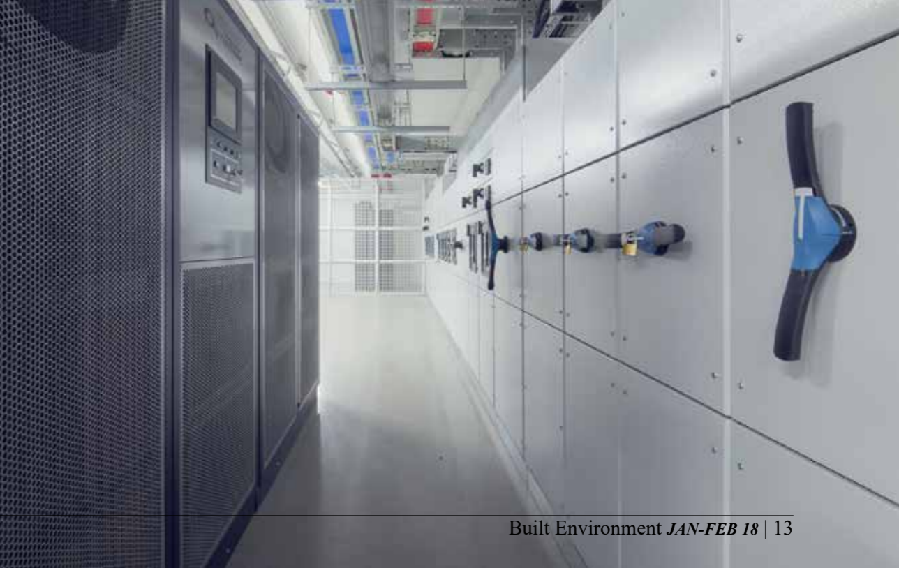
Switchgear and Uninterruptible Power Supply
