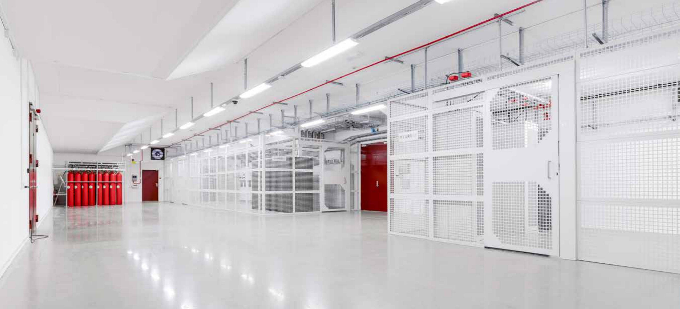
Central 'spine' of datacenter
