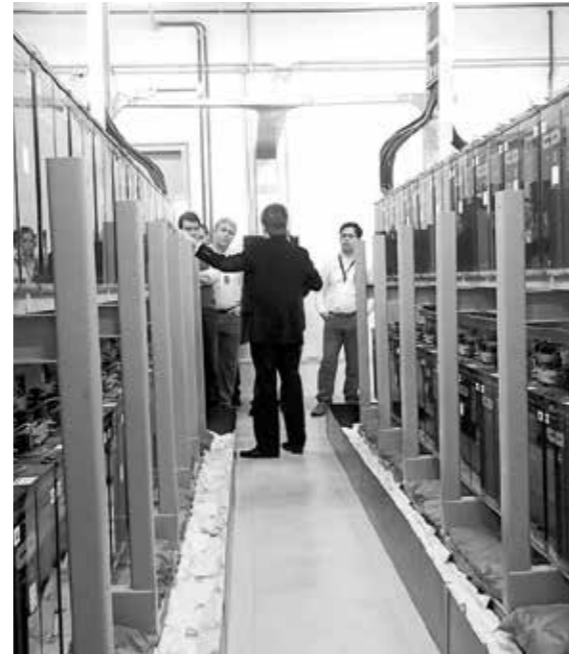
v Figure 6 Level 4 and 5 commissioning activities ensure that individual systems and the full data center ecosystem function as they were intended in the design and OPR documents.
