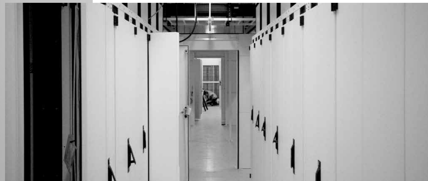
^ Figure 2 Uptime Institute notes that Level 5 commissioning includes prescribed tasks to be performed in logical order.
